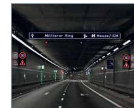
Limited variable message sign, speed limit and warning signs in a tunnel
