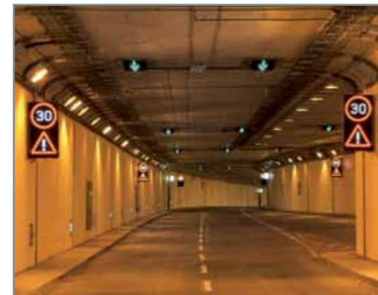
Variable message signs in tunnel, limited sign content, lane control sign (reduced total height) for mounting on tunnel ceiling Germany
